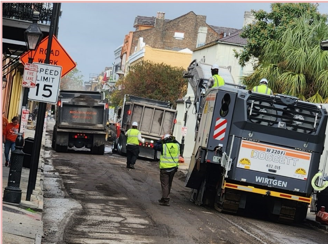
Members working with Boh Brothers Construction repaving the streets in the French Quarter preparing for the Superbowl
