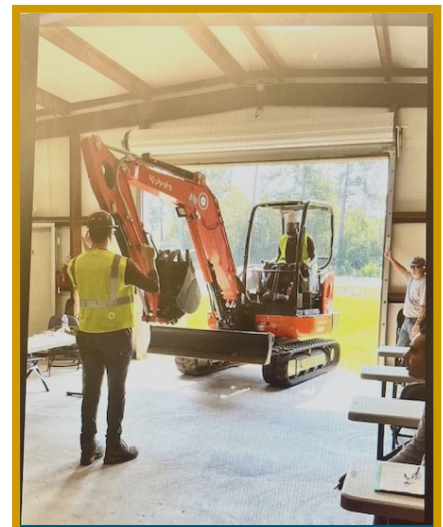
Jonathan Whittington signaling Cameron Ramadan out of shop to begin hands on excavator class
